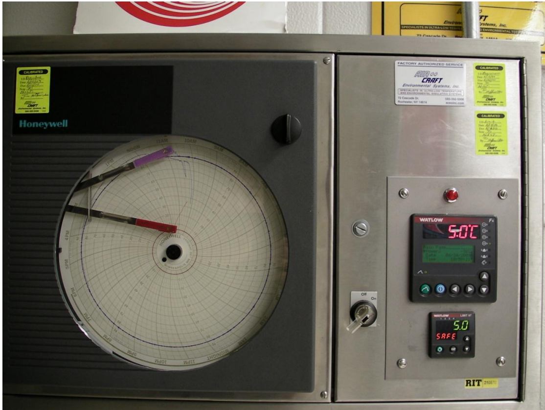
(Figure 13) Control box of environmental chamber
