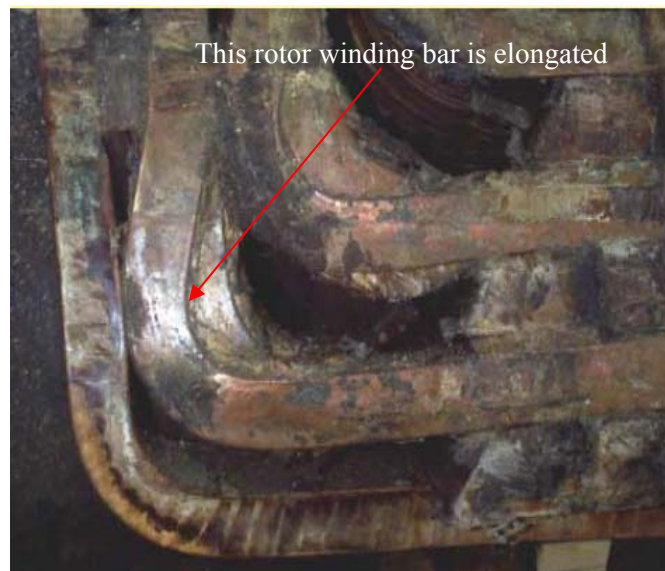
Fig. 26: An example, when Generator Rotor winding bars are elongated
