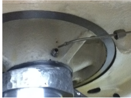
(b) Thermocouple removed from oil pump
