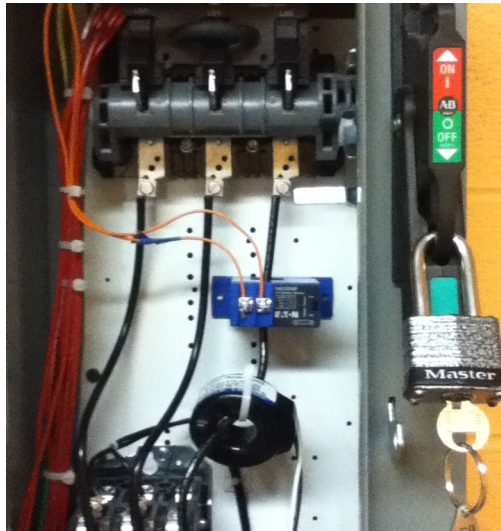
Figure 5.21: Install location for motor current sensor
