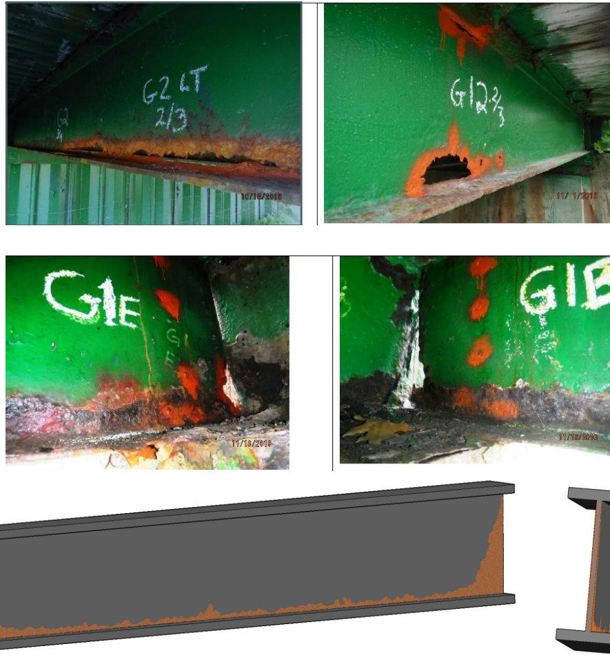
Fig. 1: Typical Steel Girder Corrosion at Web and Flange.
