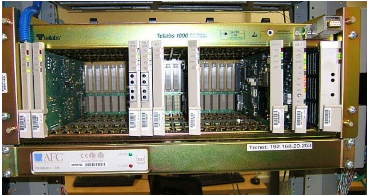
Figure 2 Optical Line Terminal
