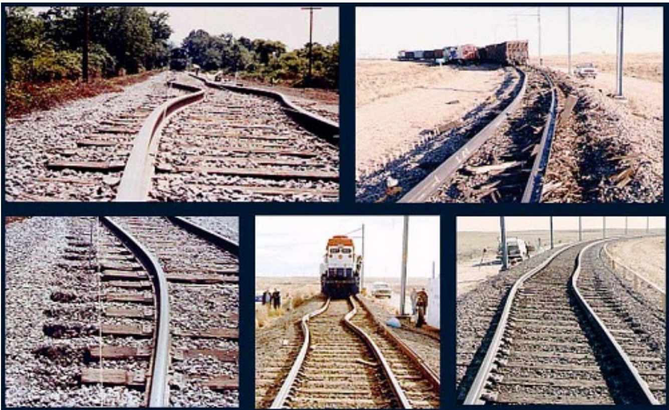
Figure 3.3.1 Buckling of railroad tracks - thermal strain (Courtesy of US Department of transportation - Volpe Center)
