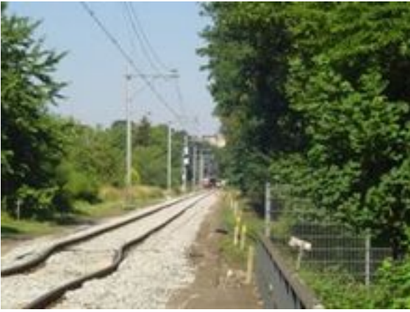
Figure 3.12.2 Buckling of tracks (Wikipedia)
