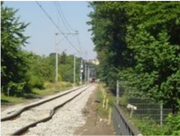
Figure 9.2 Buckling of tracks (Wikipedia)
